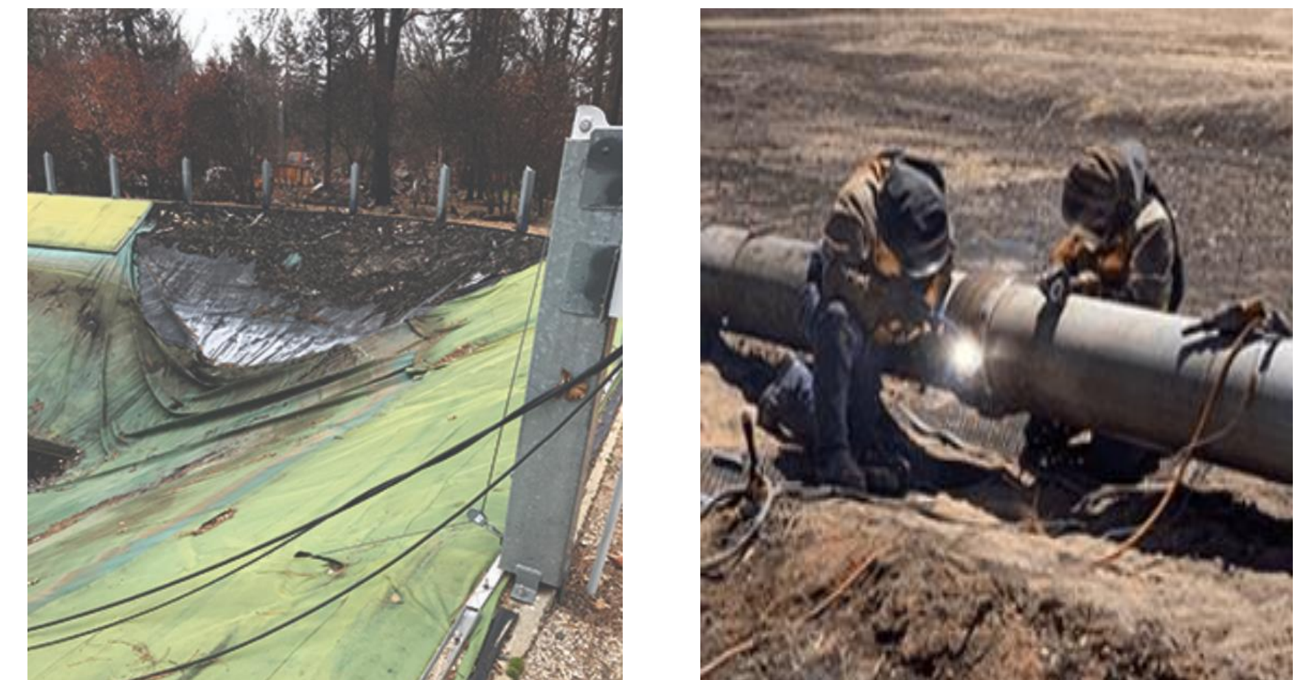
Figure 1: a) Paradise Irrigation District Service Reservoir – Nov 2018, and b) Wickepin-Dumbleyung Pipeline – Feb 2022
